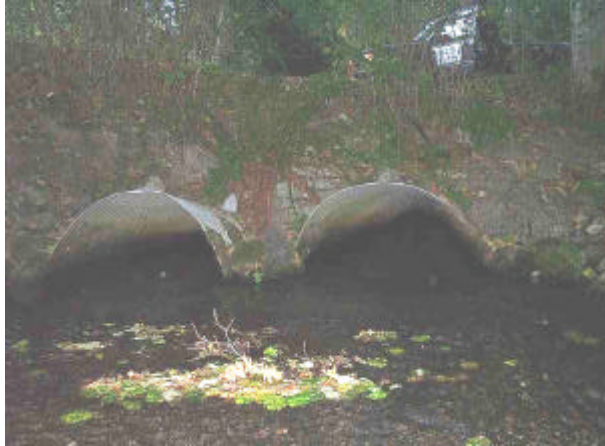
The Salazar Project on Woodland Creek will involve replacing the existing the two pipes with a Big "R" Bridge. Photo by Lance Winecka
